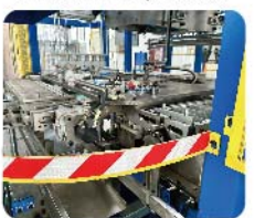
5. 铸焊工位 5. Casting and welding station
